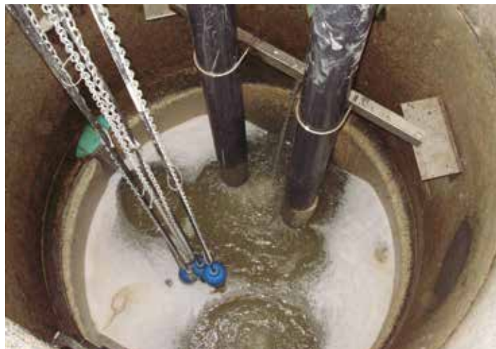
Suction pipes and float switches lead to an above-ground pump station. No pumps, mechanical equipment or electrical components exist in the wet well, eliminating the need for humans to enter the confined space for O&M.
