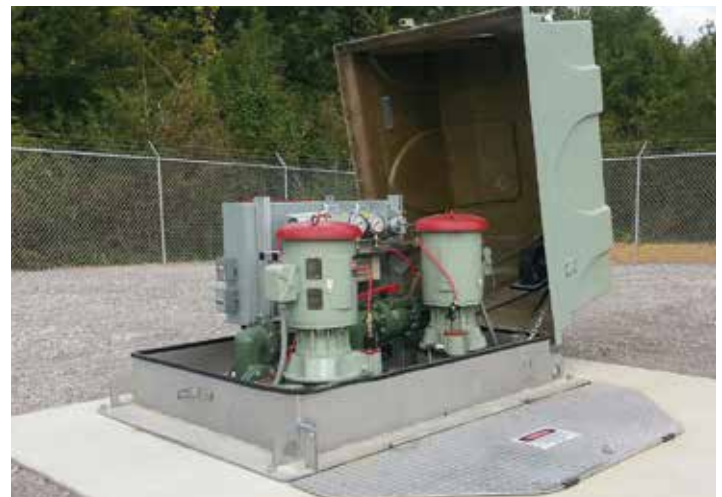
The vacuum-primed pump station, depicted (above), is one kind of above ground, prime-assisted pumping system that not only eliminates confined space requirements, but still allows for higher pump efficiencies.
