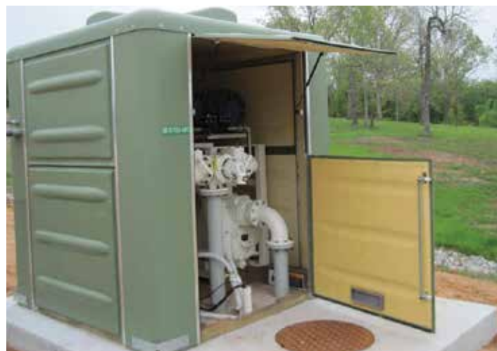
Using duplex horizontal endsuction pumps that prime with internal recirculation, the self-priming station depicted (above) includes VFDs and is accessible on each side through multiple hatches.
