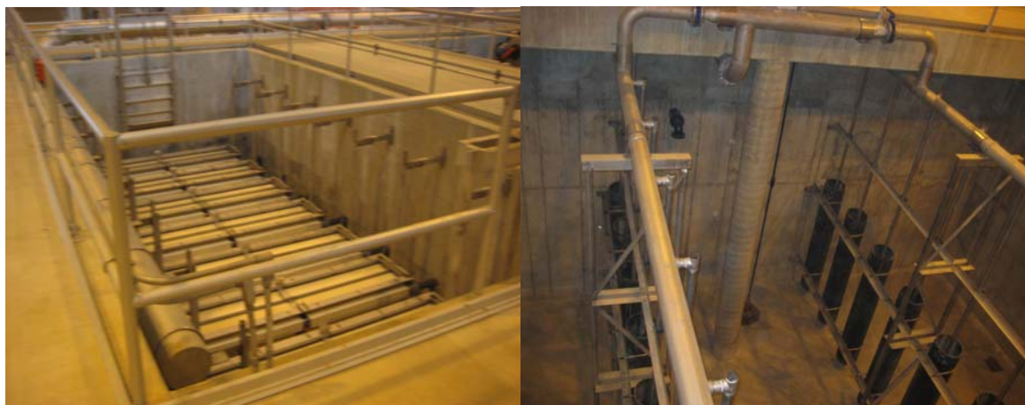
Figure 5. Union Rome WWTP Membrane Thickening Aerobic Digestion System (Membrane Thickening Tank shown on the left, Aerobic Digester shown on the right)
