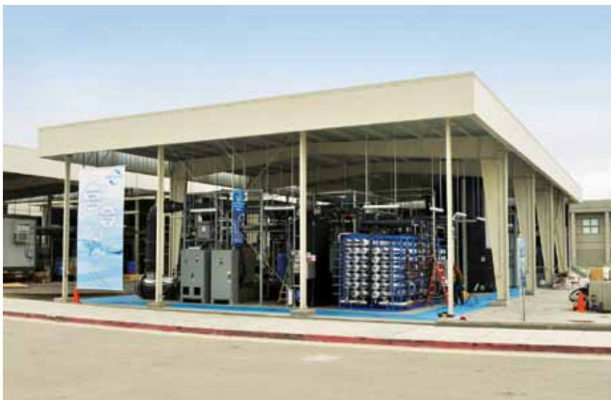
The San Diego Advanced Water Purification Facility purifies 1 million gal of recycled water to distilled water quality each day.
