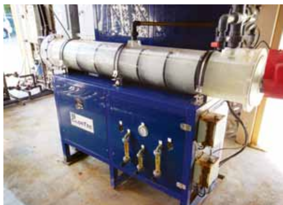
The sodium hypochlorite system
