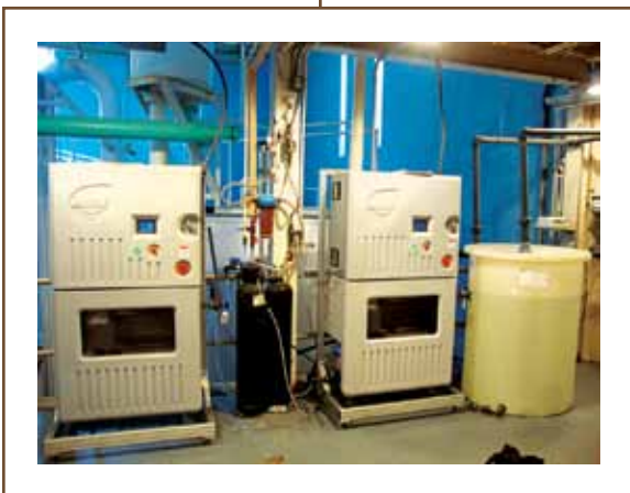
The Cedar Knox plant's electrolytic cells self-clean after 700 hours of operation, reducing maintenance needs.
