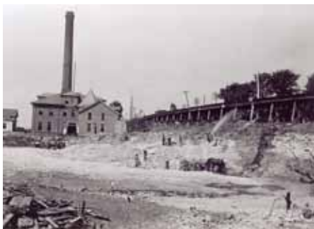
In this circa 1900 photo, workers prepare the site for construction of the original sedimentation basins at East River Station.
