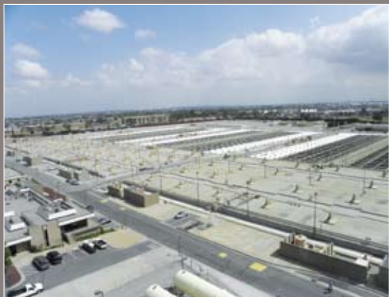
A view of the reactors and clarifiers used in the secondary treatment process.
