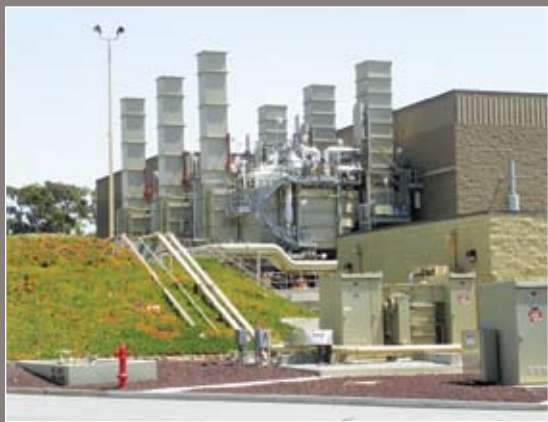
The plant's heat recovery steam generators.
