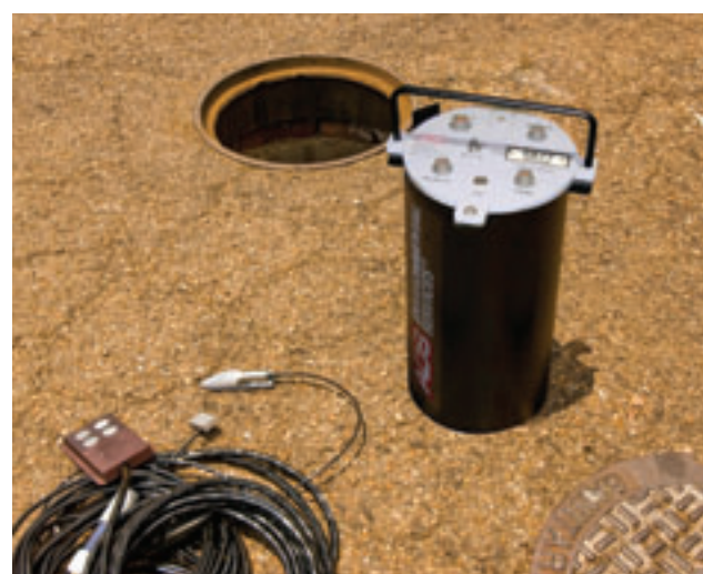
Four ADS Model 3500s with sensors were installed in 1990 and are still reporting data accurately today.
