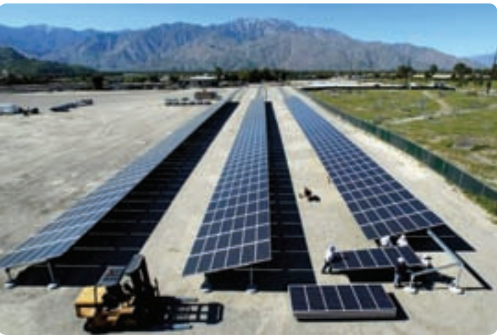
DWA has rolled out several sustainability initiatives recently, including the installation of hundreds of solar panels to provide its facilities with renewable energy.
