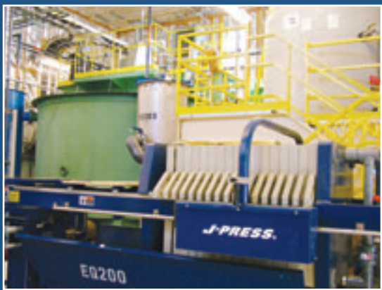
Sulphide precipitation removes cadmium and zinc from acid mine drainage at the former Wellington Oro Mine, three miles east of downtown Breckenridge, Colo.
