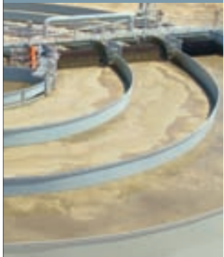
Orbal® Oxidation Ditch
