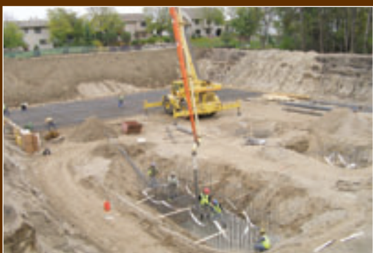
The site during the construction phase. The building took place very near residential homes, leading to increased citizen participation in the planning.
