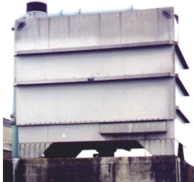
Using aerators to treat groundwaters for iron and manganese removal is effective for removing arsenic since precipitated ferric and manganic oxides readily adsorb As V.
