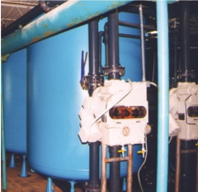
Consistent arsenic removal should be achieved using low dosages of iron or conventional dosages of alum prior to filtration.
