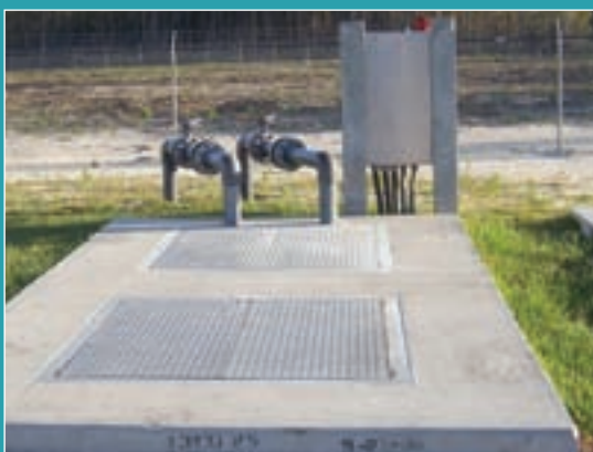
The filters gather and deposit the sand into concrete basins; city trucks vacuum it out and haul it away every six months.
