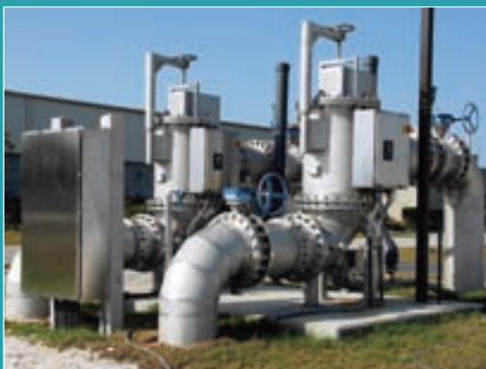
Two 9,100-gpm, multi-element, backflushing filters were installed at the Ft. Myers plant in October 2006.
