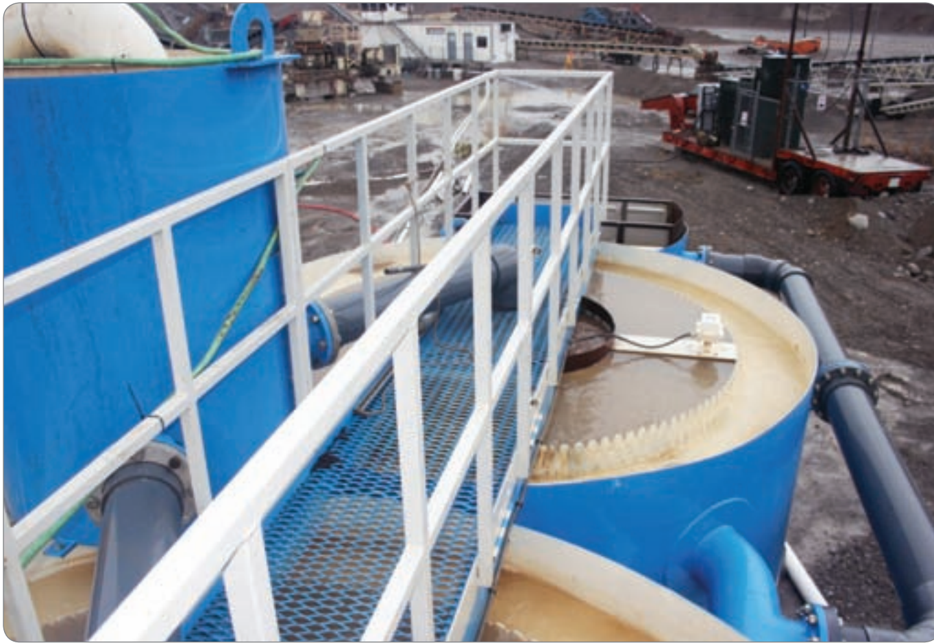
Dirty water flows from the flock tank into the two large clarifier tanks under the catwalk.
