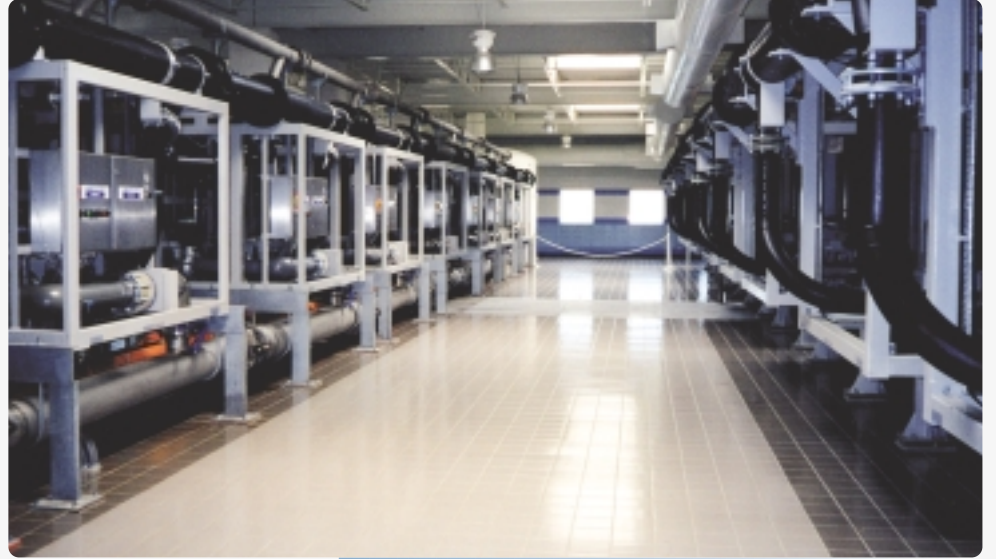
USFilter's Memcor Continuous Microfiltration (CMF) system installed at the Kenosha Water Utility treatment facility in Wisconsin.
